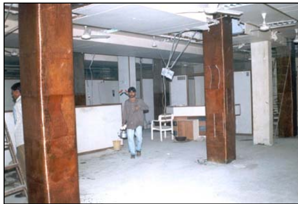
Photo 8 : Wrapping of damaged columns in a commercial building
