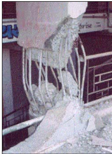
Photo 3 : Absence Of Lateral Links In Columns and Failure
