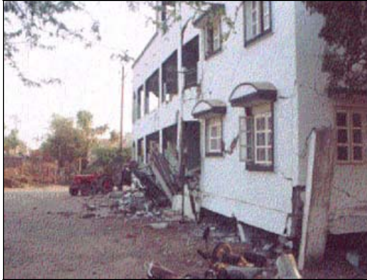
Photo 1 : Collapse of Parking story-Snapped Column
